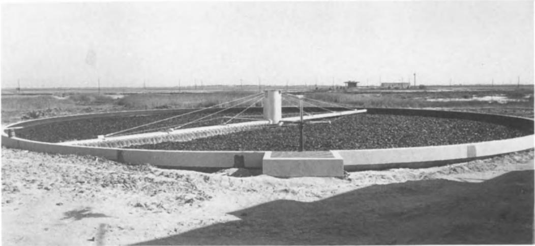
Figure 22.3. Trickling filter system used for purifying waste water from food plants as well as municipal waste systems. Courtesy of Dorr-Oliver, Inc.
